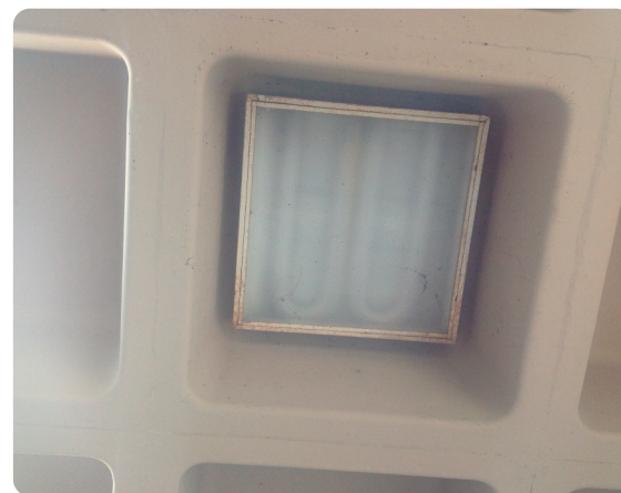
Previous rusted fluorescent troffer
