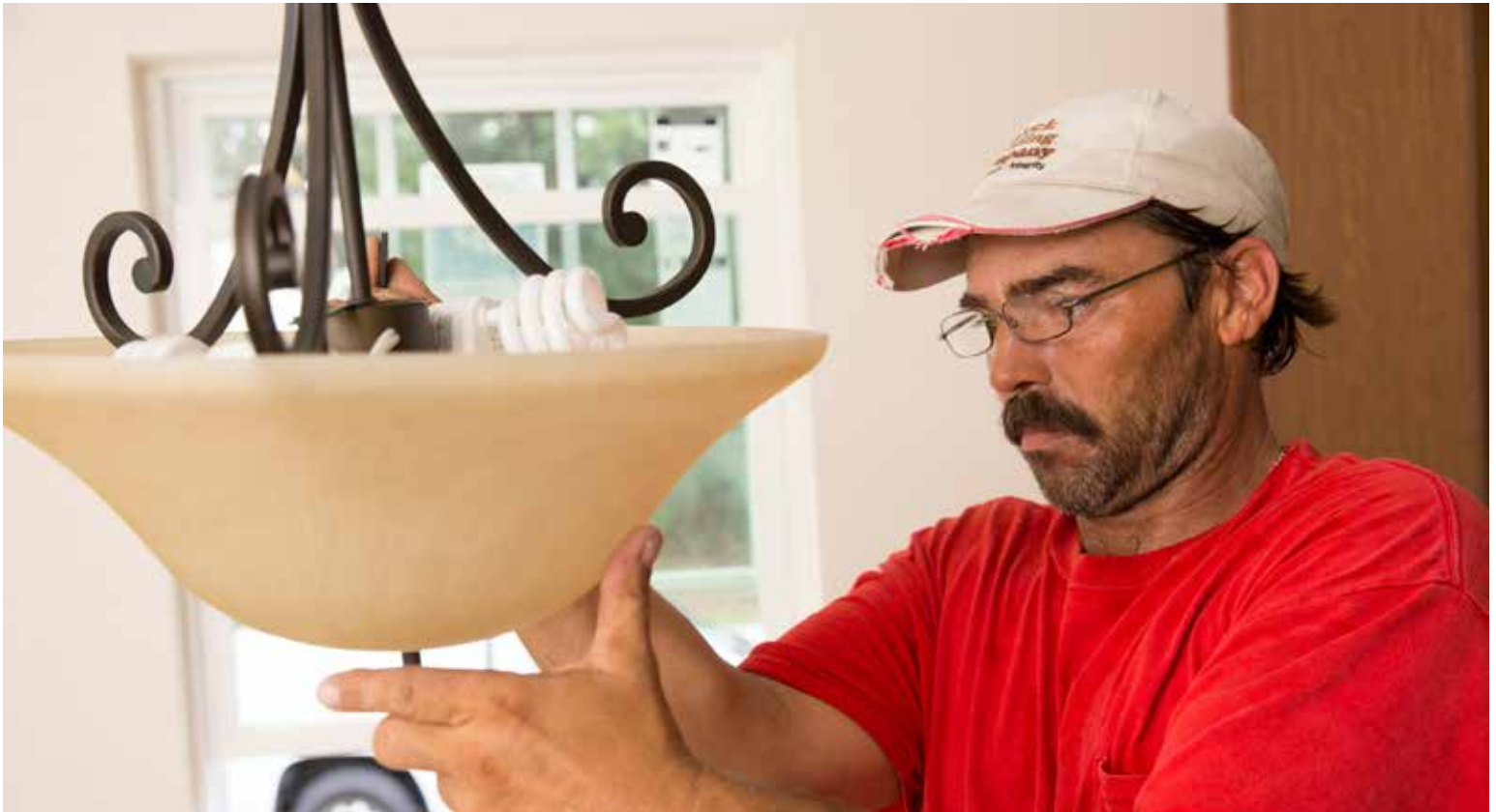
JJ Wilds, a volunteer from Hunter Electric, installs a MaxLite fixture in one of 50 newly built or renovated homes during Habitat for Humanity's Home Builders Blitz in Jacksonville, Florida, in June 2014.
