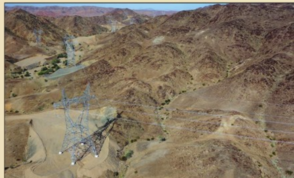
The 110-mile HANG2 transmission line is now only the second power line to connect Phoenix to Yuma.
